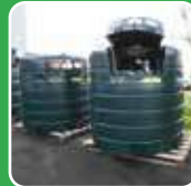
LOCAL DE STOCKAGE FUEL
